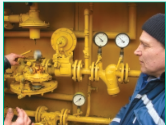
Measuring methane emissions at a gas distribution centre after installing new equipment
